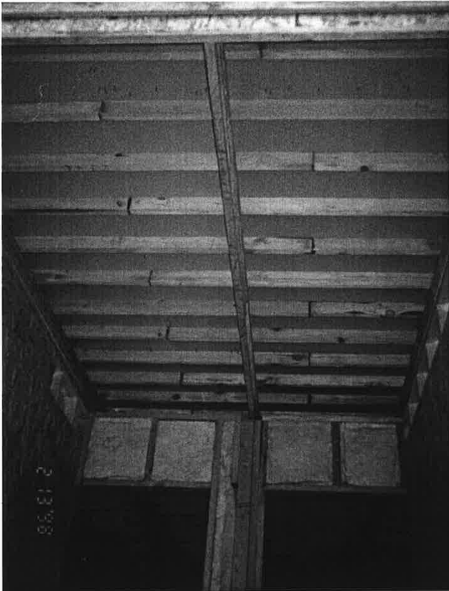
Figure 25. Incorrect I-joist spacing and improper ceiling joists.
