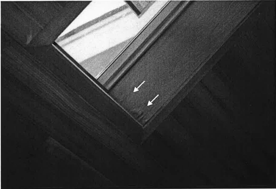
Figure 147. Damage due to poor skylight installation.
