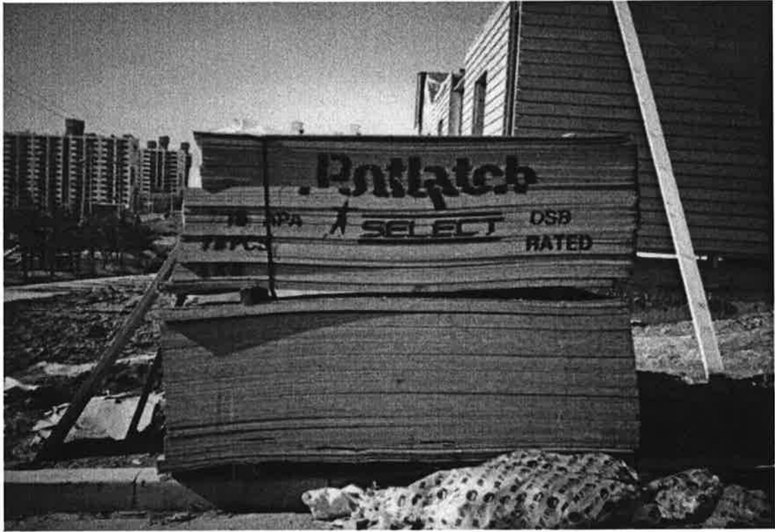
Figure 26. Improper site storage of OSB panels.
