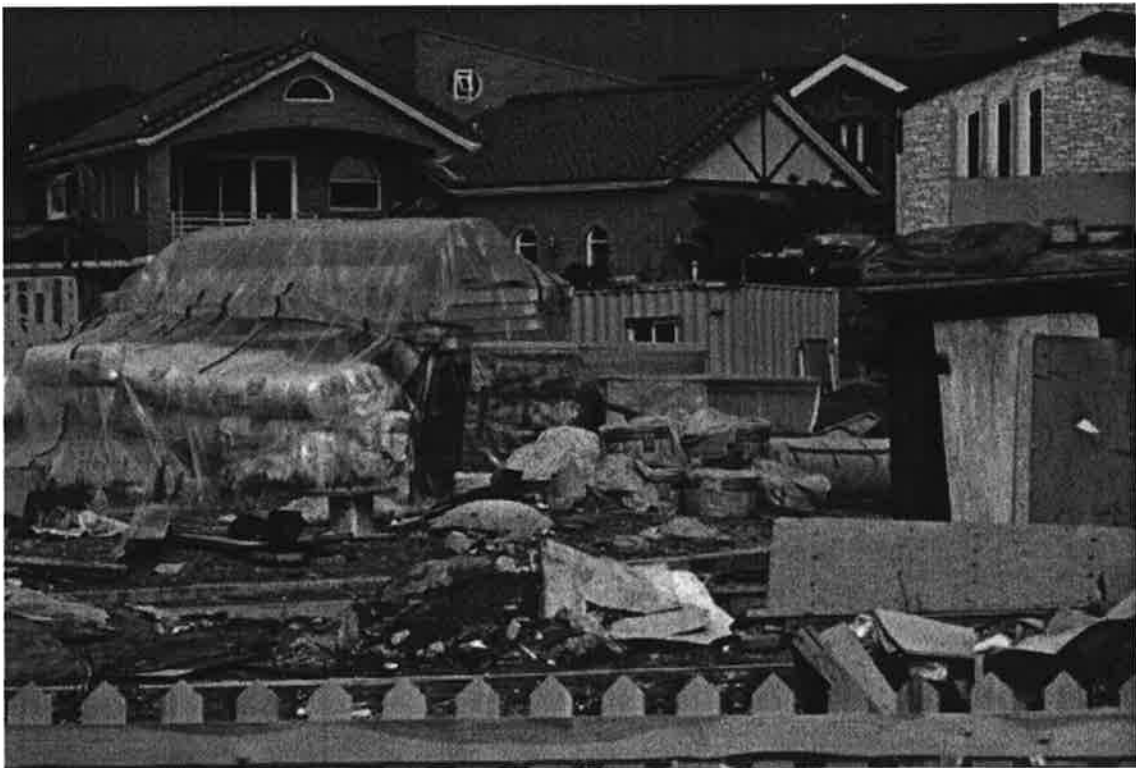
Figure 27. Inadequate site storage of building materials.
