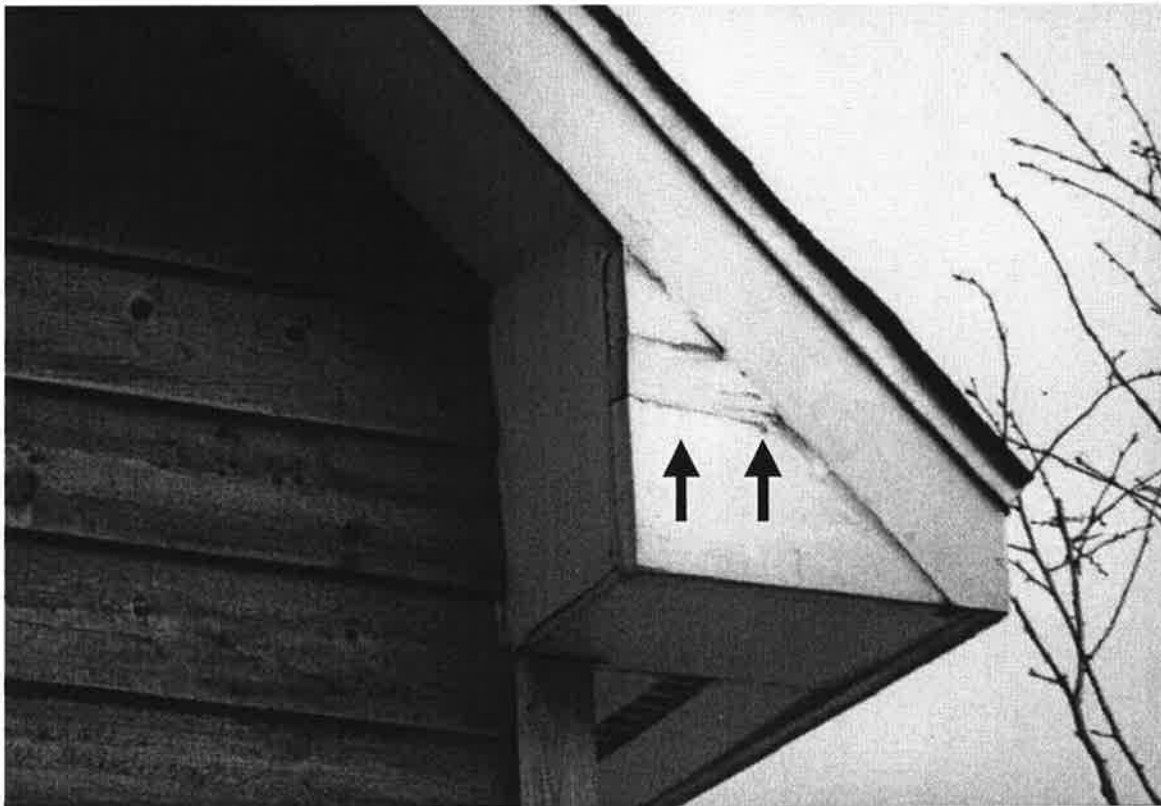
Figure 13. Product quality and paint failure.
